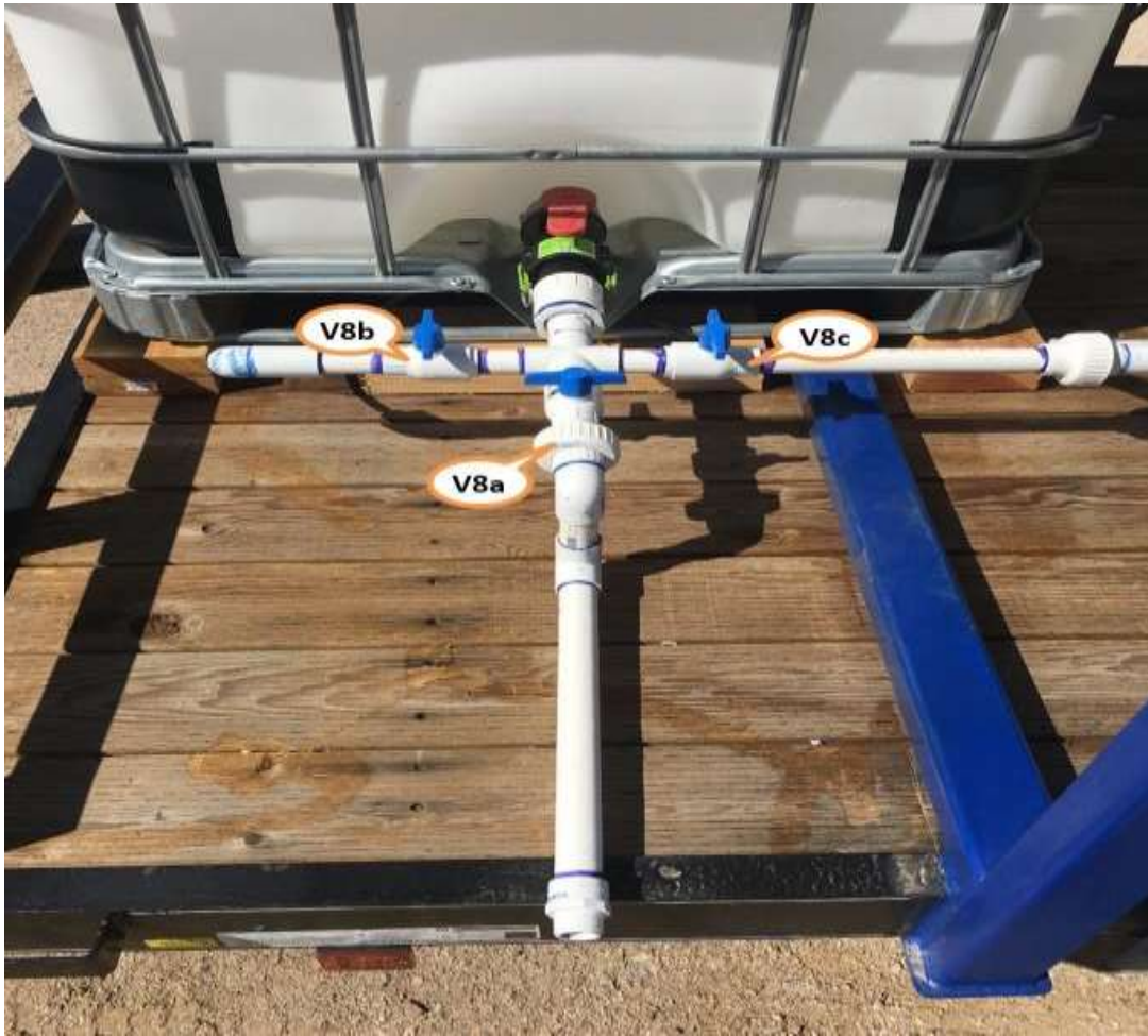
Figure 8. Bottom exit of the finished water tank. From here water can be withdrawn or released by gravity for (i) direct use—lower pipe with exit shown, (ii) UV treatment prior to potable use (pipe at left) or (iii) membrane rinsing during system shut-down (pipe at right). Corresponding valves are V8a, V8b and V8c, as shown. Valve V8d can remain open.
