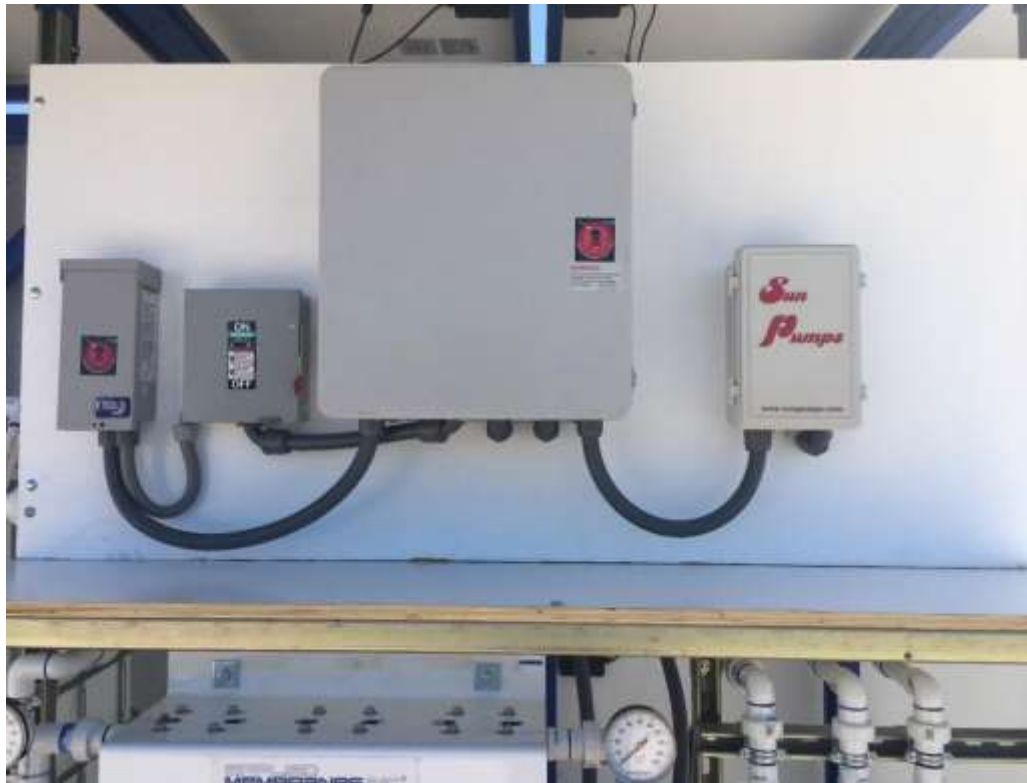
Figure 6a. Electrical control boxes located above the prefilter array. Individual boxes and interior switches are shown in Figures 6(b-e).
