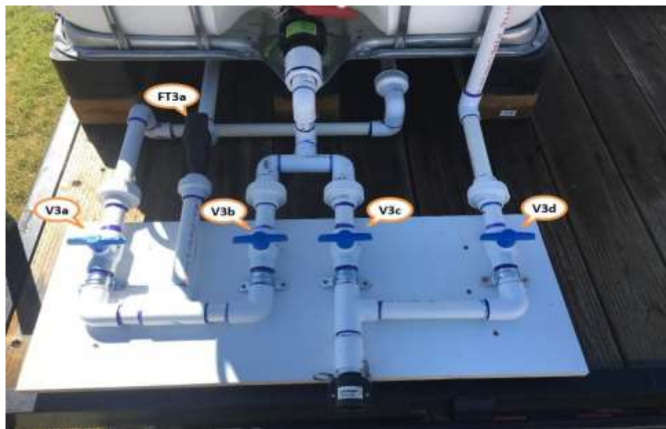
Figure 3. Raw water feed manifold. In normal operation, water is drawn from the raw water tank (partially visible atop the figure), through the red valve (partially shown) and valve V3b, past the black screening device at FT3a and then back (under the tank) to the pump (Figure 4).
