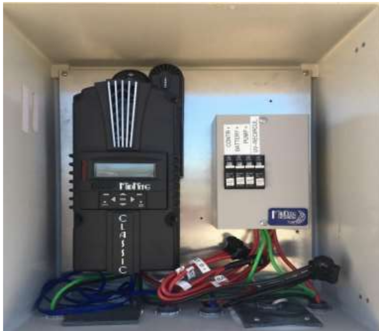
Figure 6d. Interior of the charge control box. During normal operation, the first three circuit breakers should be in the “on” position, as shown. The fourth switch should be off unless the finished water is being disinfected using the UV lamp—later section. The charge controller is at left.
