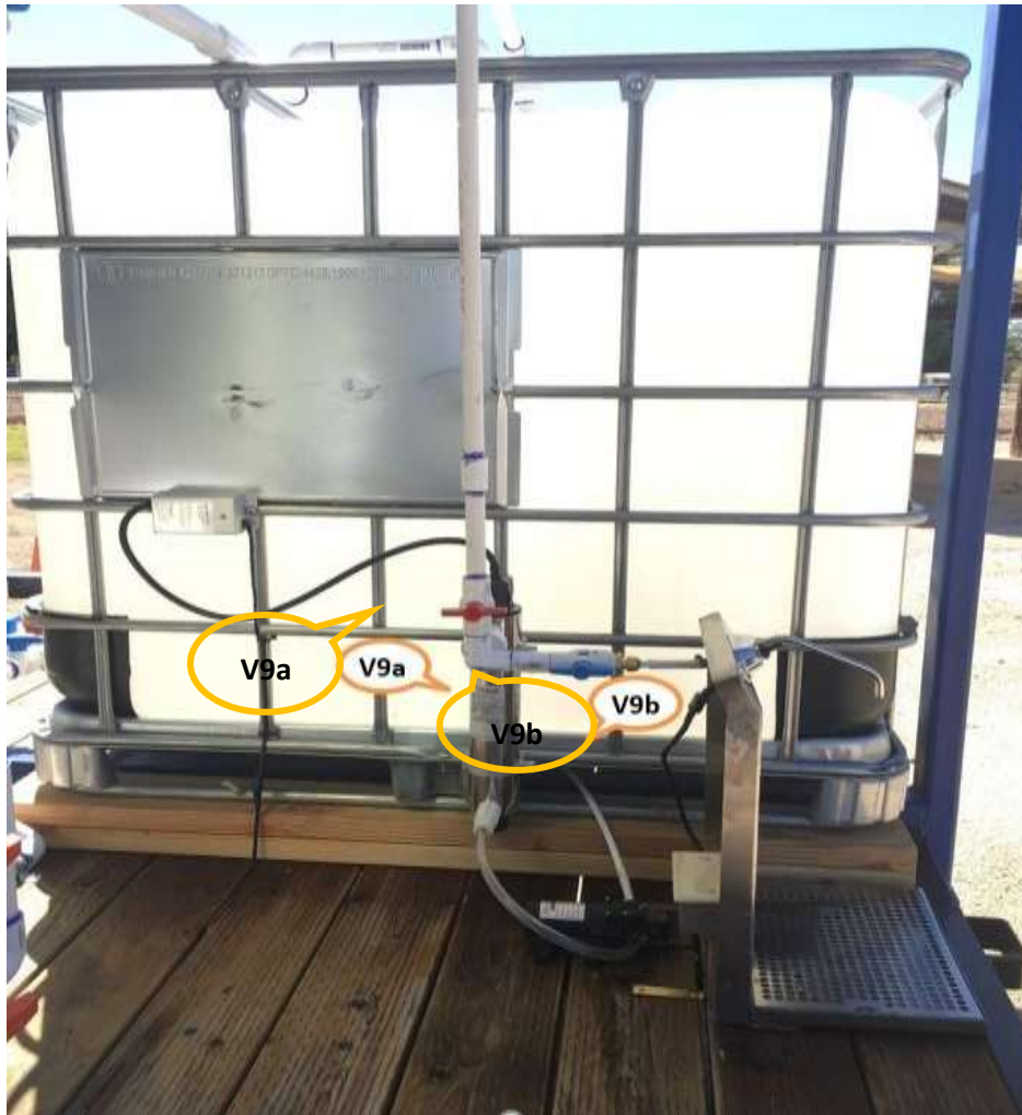
Figure 9. Ultraviolet disinfection system. The system is located adjacent to the finished water tank. UV treatment can be provided via two means: Single pass operation for disinfection prior to delivery of water from the stainless steel spout at right or continuous re-purification with water taken from and returned to the finished water tank.
