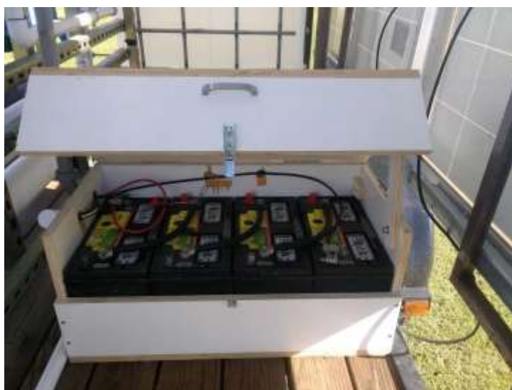
Figure 7. Batteries (four, 12V lead/acetate) and battery containment box. The four batteries shown are connected in series to provide a working voltage of 48-52V, depending on battery state of charge.
