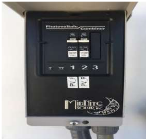
Figure 6c. Left-most of four electrical boxes in Figure 6a. To operate the pump, circuit breakers should be positioned as follows—nos. 1 and 2 “on”.
