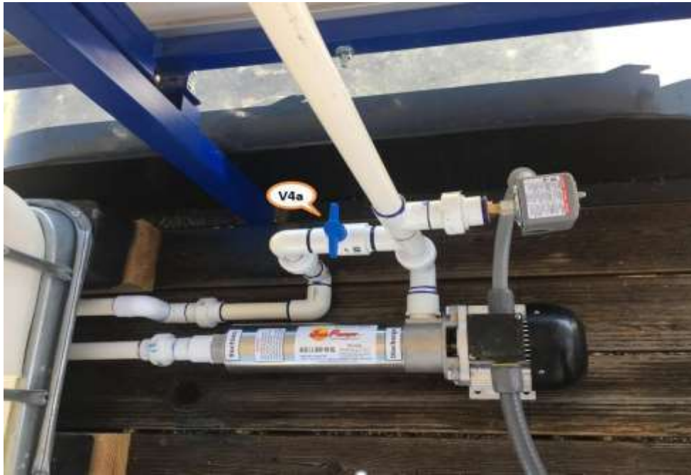
Figure 4. View of pump and piping behind the (blue) prefiltration units. V4a should be closed during normal operation to prevent pumped water from simply returning to the feedwater tank or to discharge without passing through the prefilter or membrane arrays.
