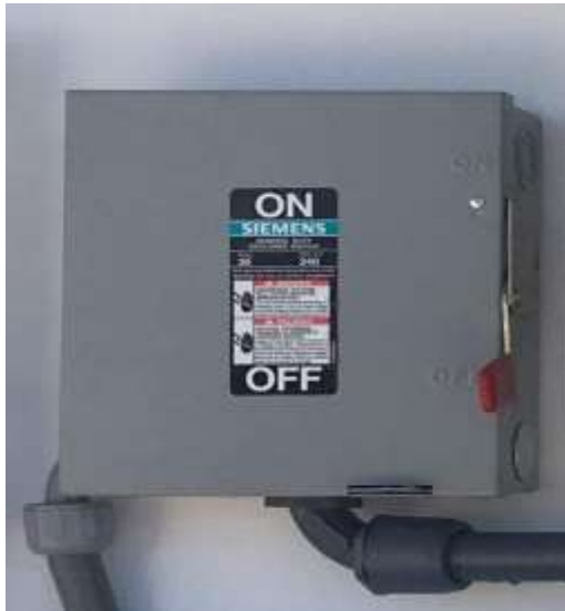
Figure 6b. Main breaker box with lever in the “off” position. The solar array is disconnected from other elements of the power train.
